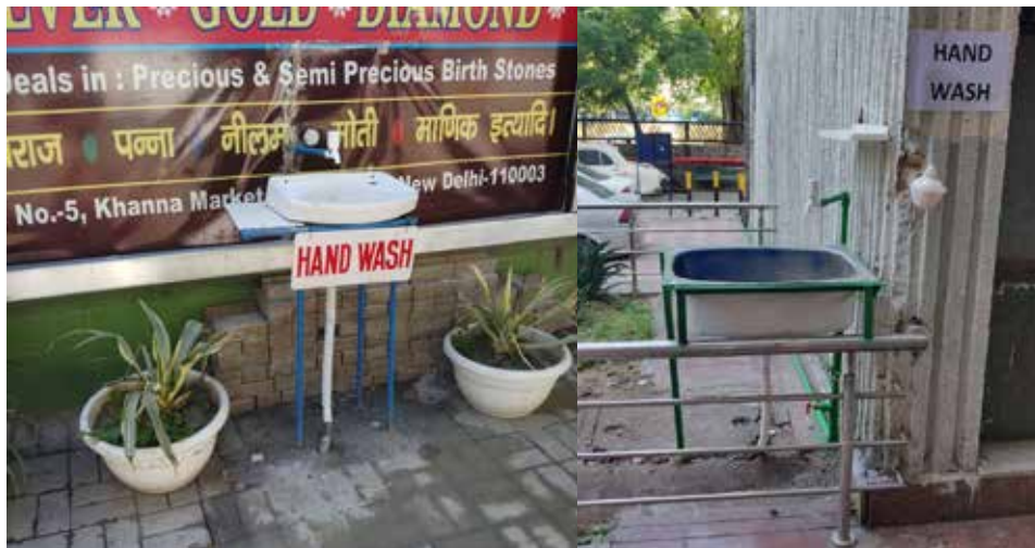
Hand wash facility at Khan Market, Palika Bhavan
